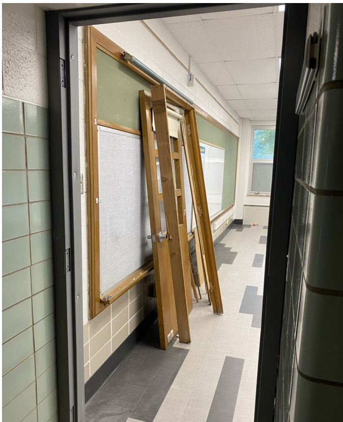
Wood door & frame getting replaced by a metal door & frame at Wall Elementary School.
