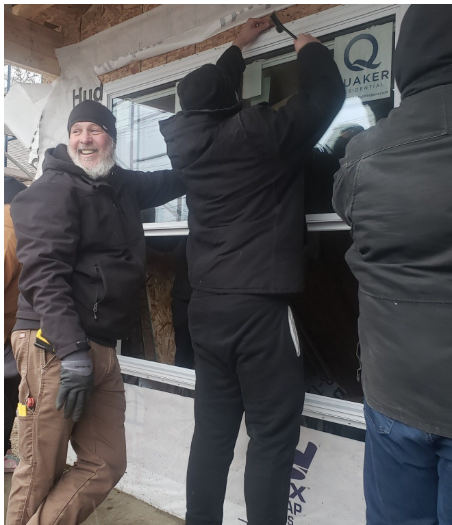
Wally Wheeler mentors CTE students as they build a house in coordination with the Sturgis Neighborhood Program in Sturgis.
